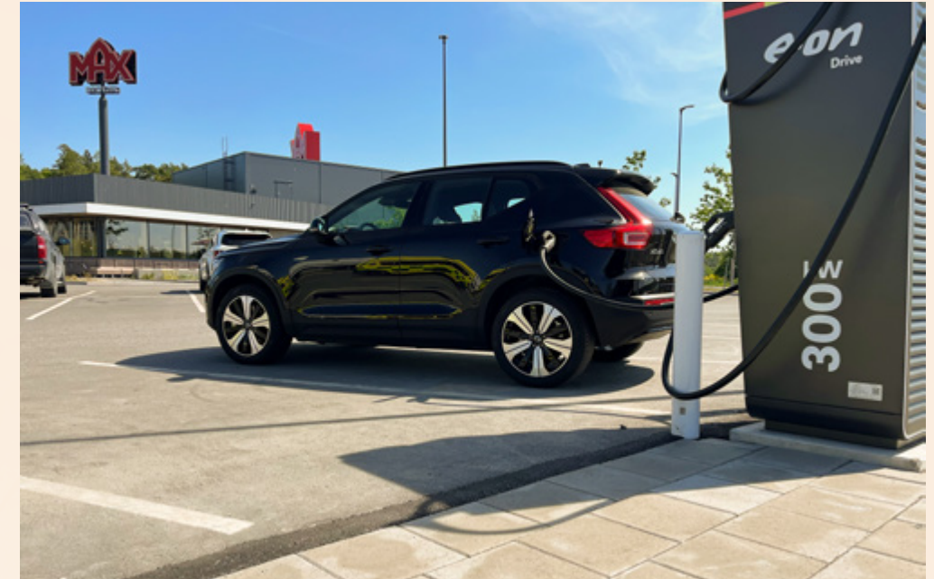
One of 254 electric car charging points at a MAX restaurant in Sweden.
